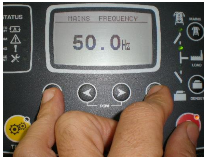
Hold pressed OFF , LAMP TEST and ALARM MUTE
